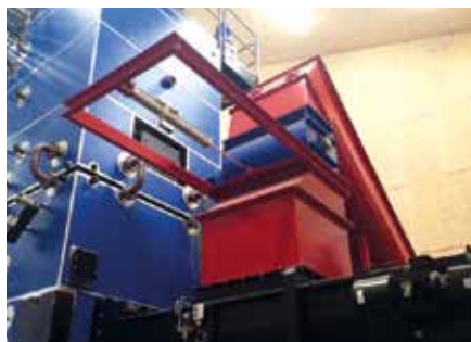
Straw burner feeding system and knife gate for back fire protection.
